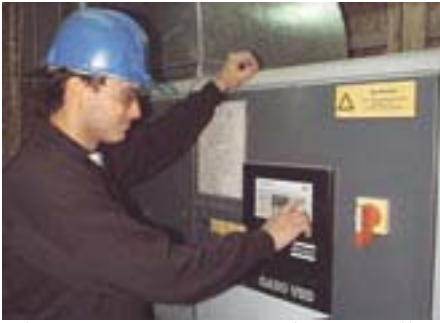
The new VSD compressor has virtually eliminated production downtime on the air nailers used to assemble fence panels. Nail placement is also more uniform.
