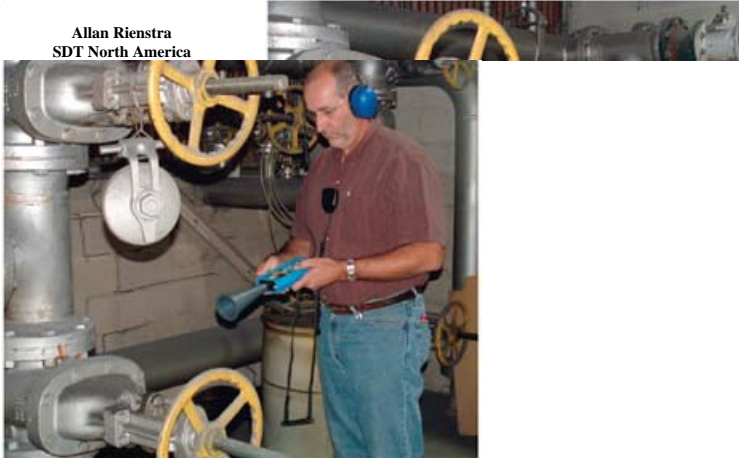
Fig. 1. Maintenance foreman Randy Treadway, of the AFG Industries plant, Greenland, TN, recently was certified in Ultrasonic Analysis by SDT North America. Here he demonstrates the use of the SDT 170MD to detect air leaks.
